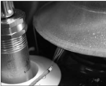
Figure 34 - Test the air supply and vent to make sure the water heater has adequate air and is venting properly.
